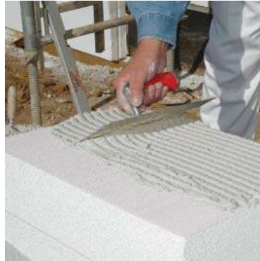
Apply over full surface with toothed trowel (10 or 12 mm teeth) results in adhesive surface of at least 70%.
